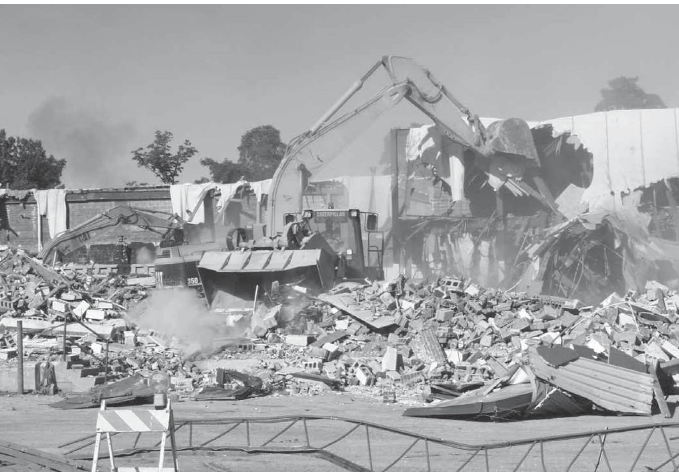
Partial demolition of the “old freezer building” on Front Street, 2001. The building debris was used to raise the elevation of the site.
